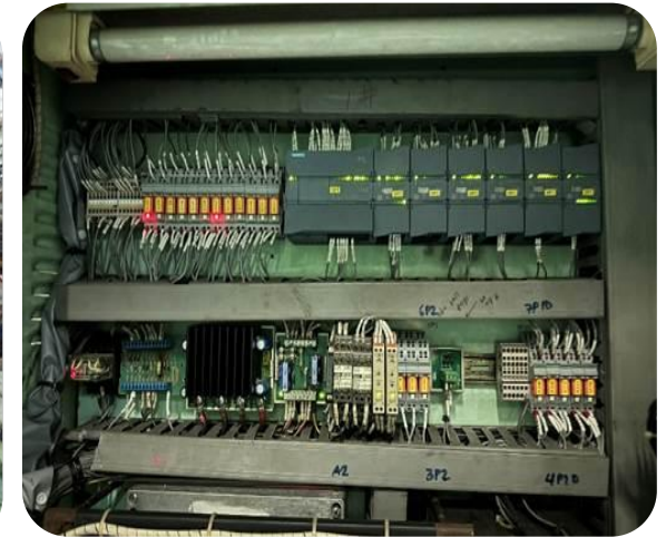
ENGINE PLC MODIFICATION
